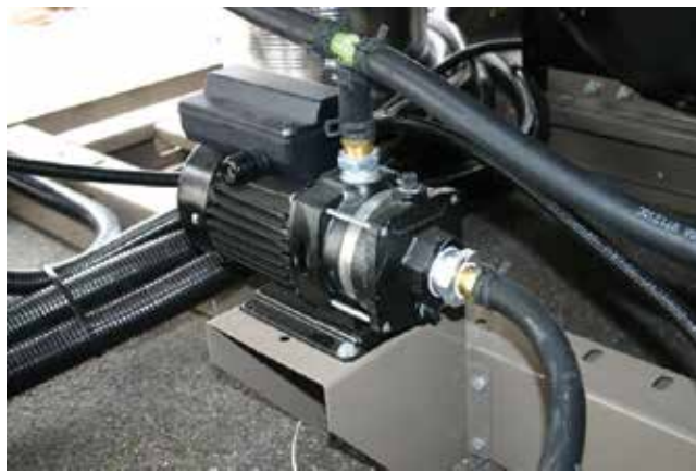
FIGURE 103 - VSD GLYCOL PUMP
