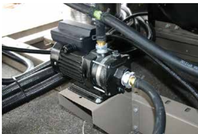
FIGURE 106 - VSD GLYCOL PUMP
