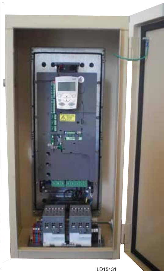
FIGURE 103 - INVERTER WITH KEYPAD AND DISPLAY INSTALLED
