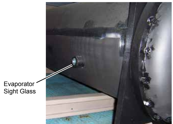
FIGURE 8 - EVAPORATOR SIGHT GLASS
