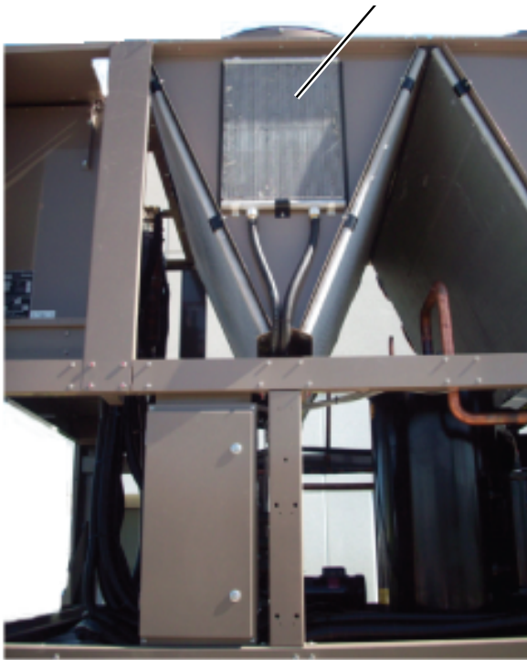
VSD COOLING - GLYCOL COIL
