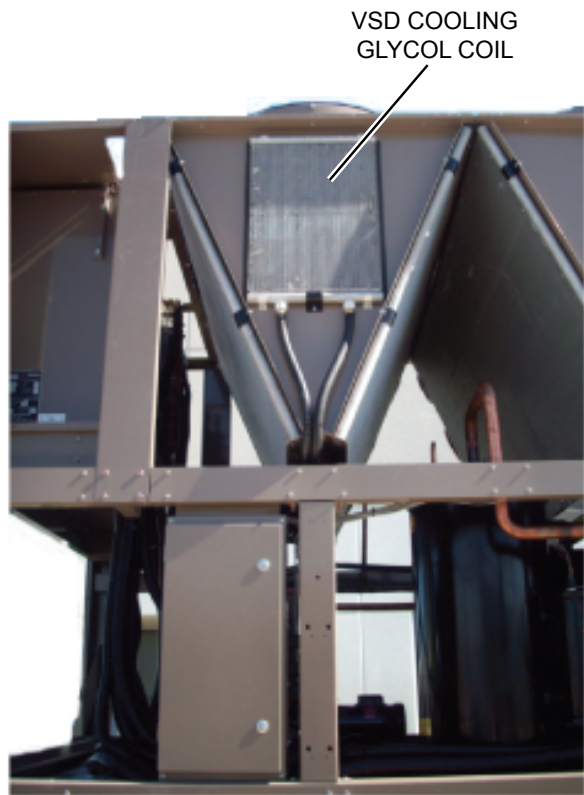
FIGURE 24 - GLYCOL COOLING COIL
