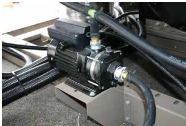
FIGURE 104 - VSD GLYCOL PUMP
