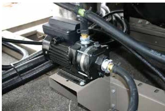
FIGURE 105 - VSD GLYCOL PUMP
