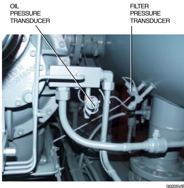
FIG. 18 – OIL AND FILTER PRESSURE TRANSDUCERS
