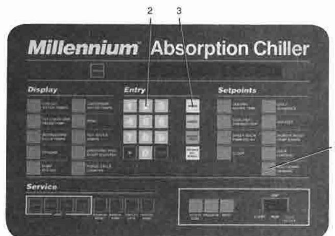
FIG. 11 - KEYPAD - PROGRAMMING "PULL DOWN DEMAND" SETPOINT
