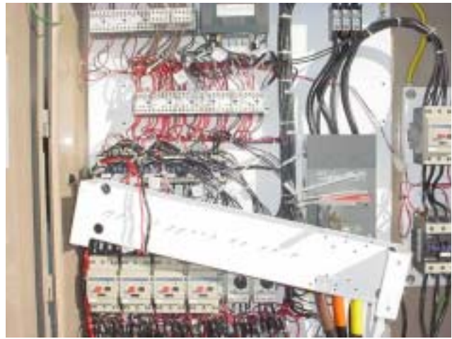
FIG. 4 - FUSE PANEL REMOVED
