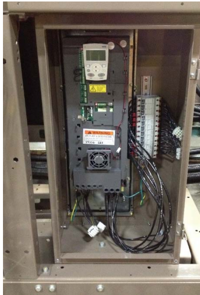
Fan inverter in enclosure
