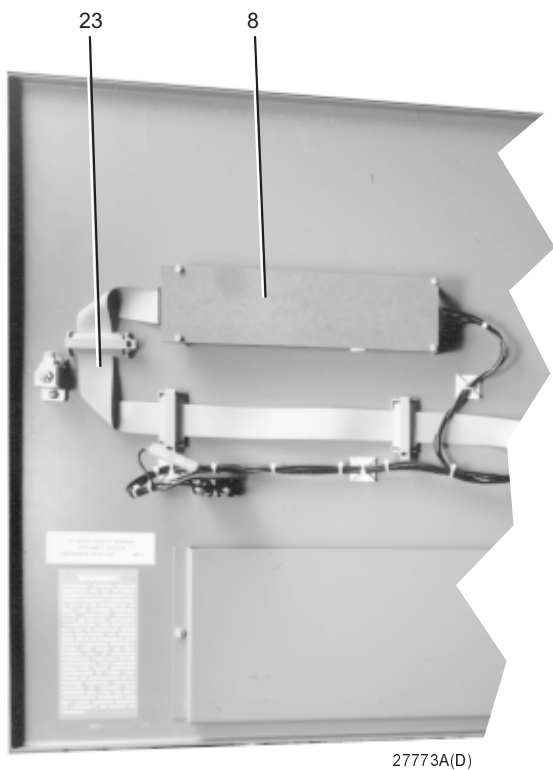
FIG. 2 – YORK MICRO PANEL CONTROL CENTER (DOOR OPENED)
