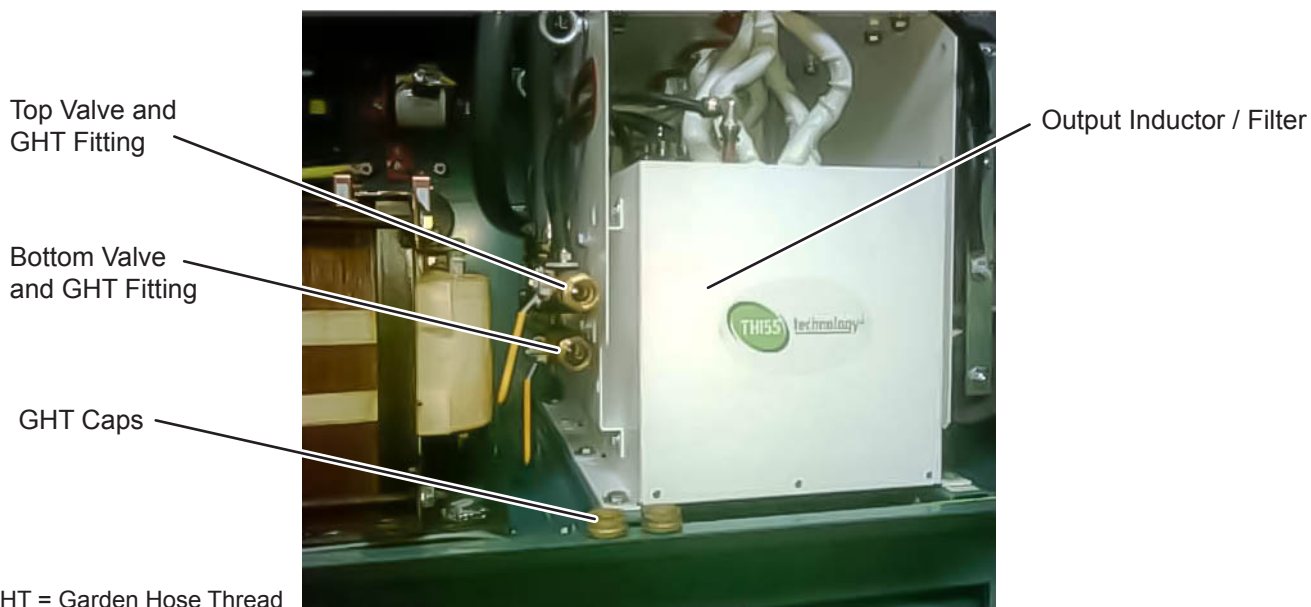
FIGURE 1 - INSIDE OF VSD CABINET
