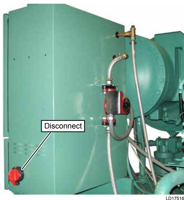
FIGURE 26 - POWER PANEL BATTERY DISCONNECT SWITCH
