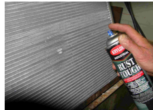
Protect against corrosion
