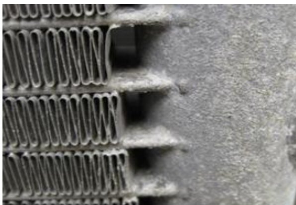
FIGURE 7 – Typical MCHX with Visible Flux Residue
