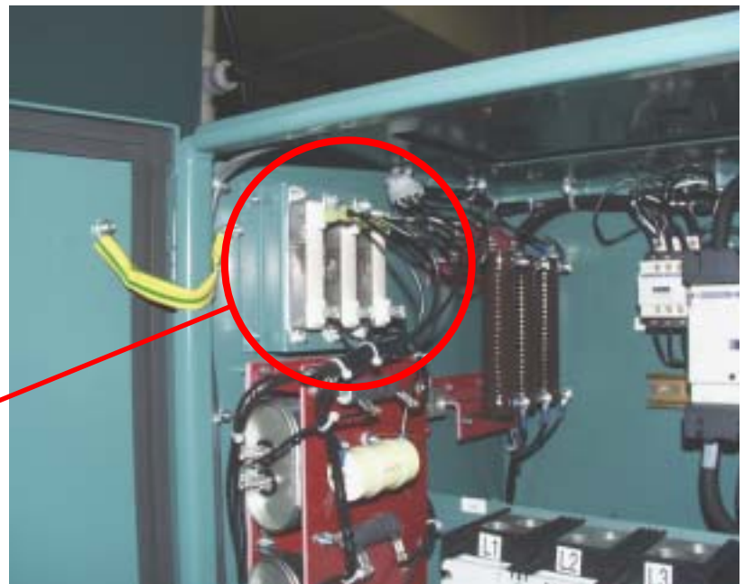
FIG.1 - LOCATION OF TRAP FILTER POWER RESISTORS
