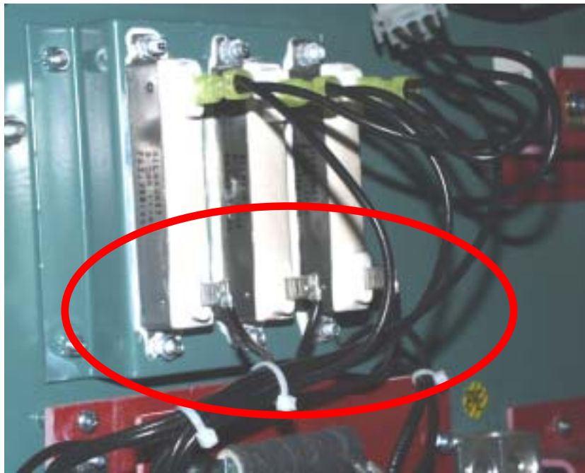
FIG. 3 - WIRE ROUTING IS CORRECT ON THE BOTTOM OF THE TRAP FILTER POWER RESISTORS
