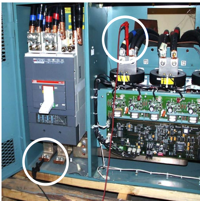
Figure 3 above shows the location of the voltage probes to measure the AC voltage from L1 – T1. Repeat this measurement for L2 – T2, and L3 – T3.
