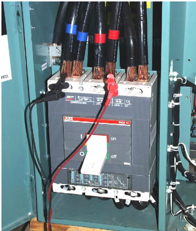
Figure 1 above shows the location of voltage probes to measure phase to phase voltage. Repeat this measurement for the other 2 phases.
