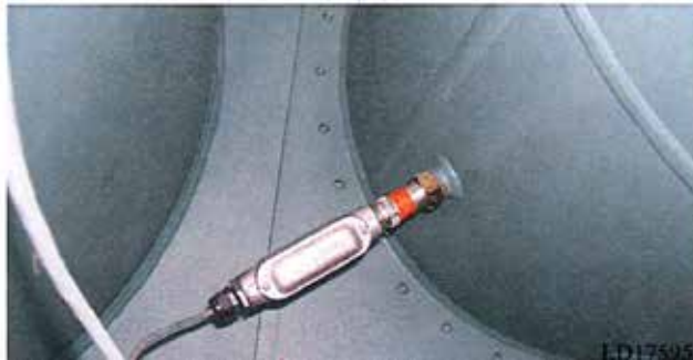
FIGURE 1 - REFRIGERANT LEVEL SENSOR
