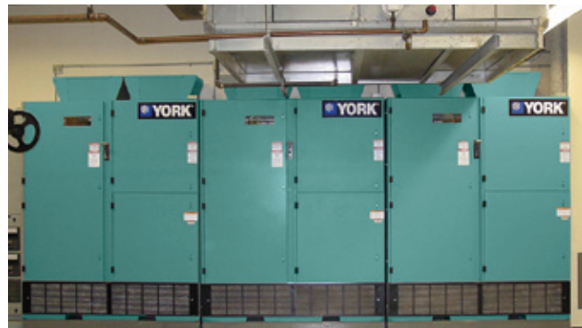
The medium-voltage OptiSpeed drives fit back into the space once occupied by solid-state starters.
