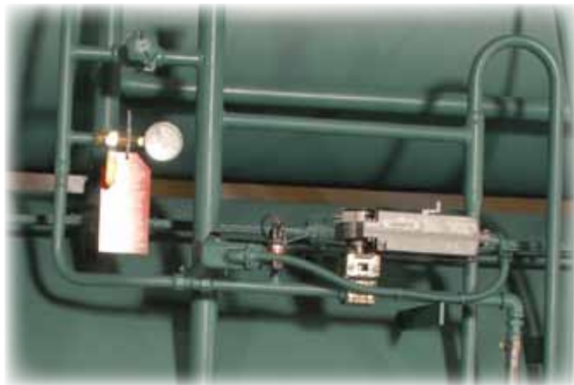
Factory Installed Gauge
