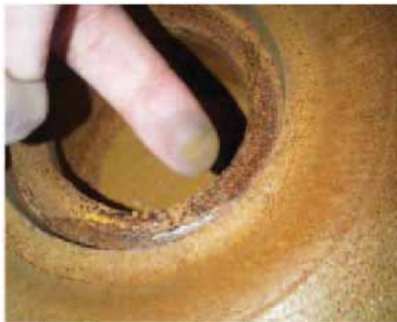
FIGURE 2 - CORRODED VOLUTE CLOSE-UP
