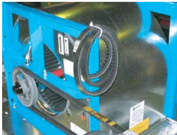
SPARE FAN BELT (Attached to Fan)
