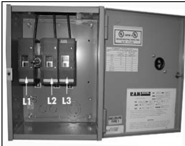
Incoming Power Drive w/Fused Disconnect
