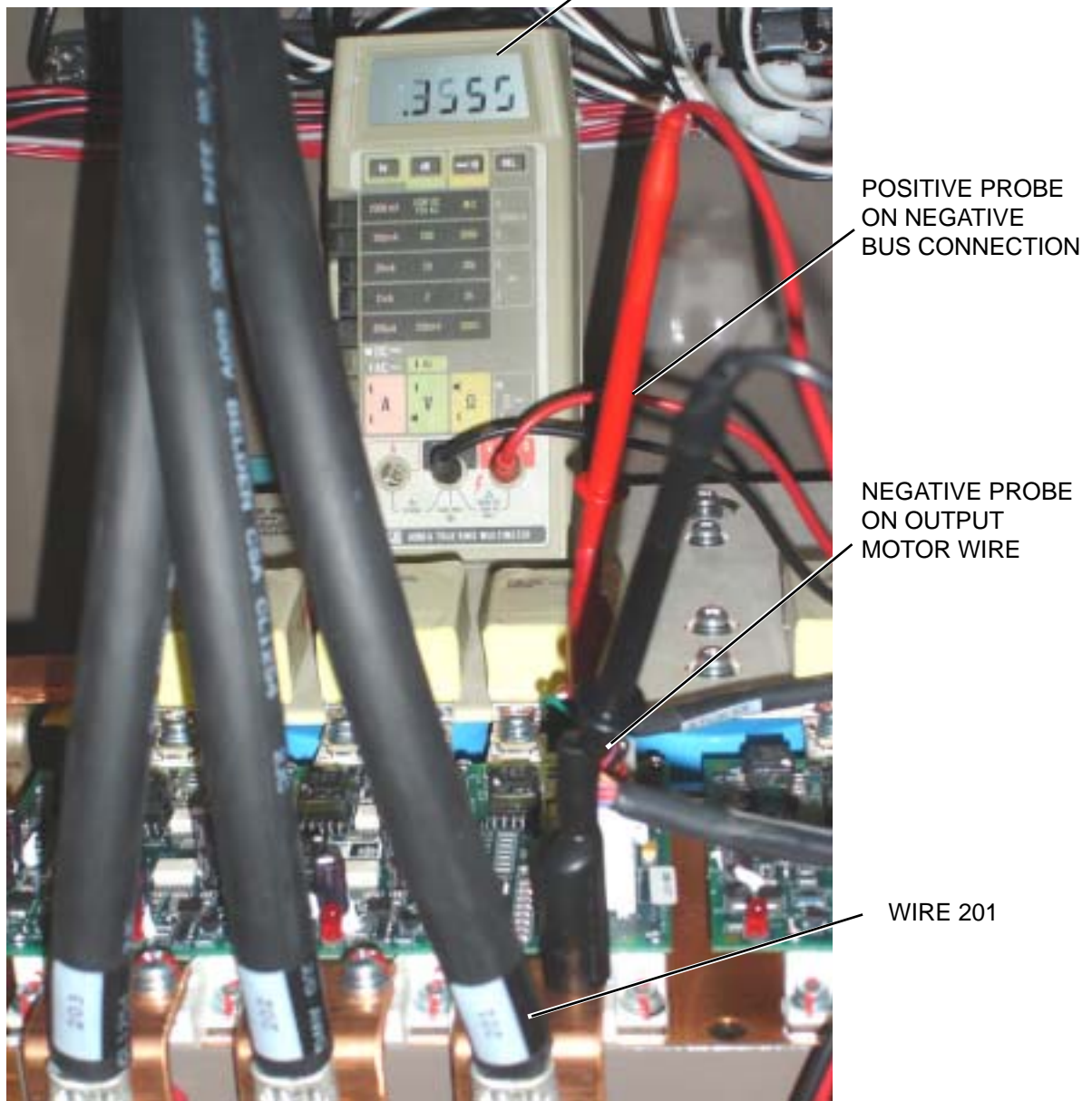
FIG. 5 – IGBT MODULE VERIFICATION
