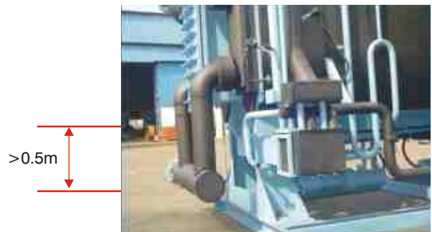
NPSH (R) maintained
