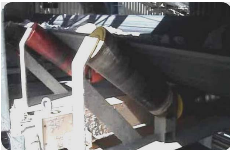
Figure 11 - 1. Conveyor Idler Rollers.
