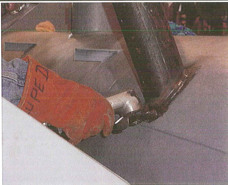
Clean and stamp welds. Allow welds to cool prior to proceeding. All welds to be coated with primer.
