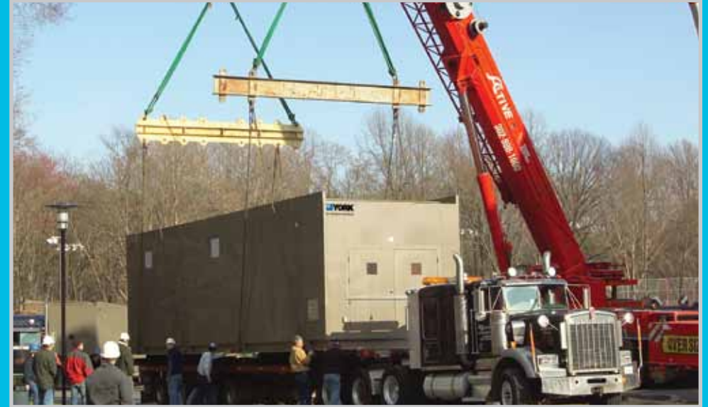
Modular Central Plants greatly reduce project lead times because plant production occurs concurrently with the associated major components and on-site work.
