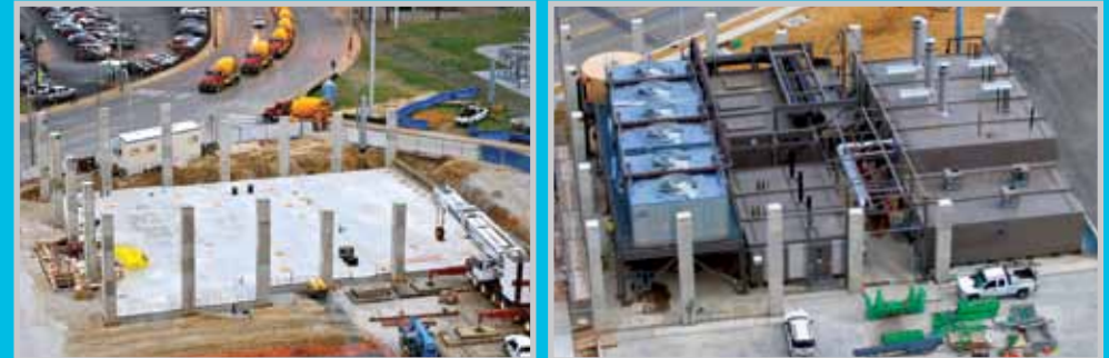
At a Le Bonheur Children's Hospital, an empty 12,000-square-foot pad was turned into a Modular Central Plant in just a fraction of the time it would have taken using traditional construction methods.
