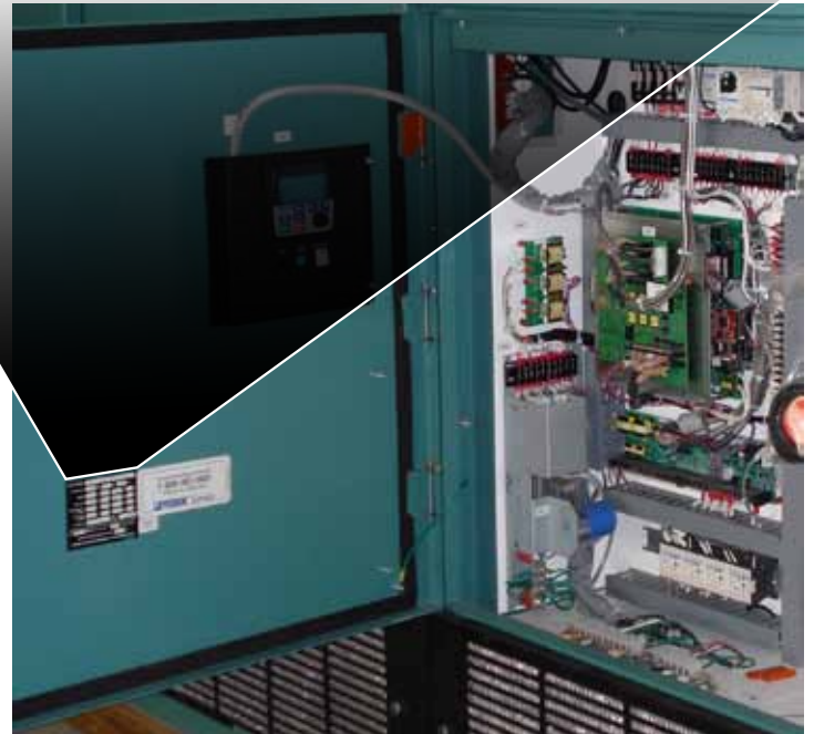
LOW VOLTAGE COMPARTMENT
