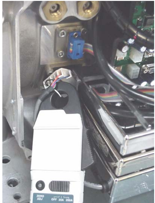
Figure 4-54 Measuring the Bearing Current Output
