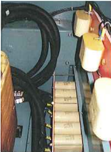
The 20 kHz Trap is re-installed into the VSD
