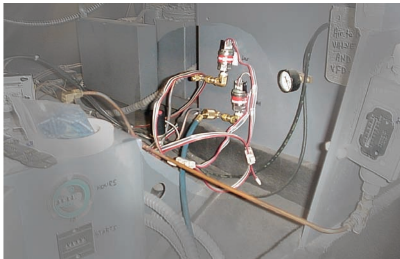
Figure 9. Pressure transducers mounted outside of control cabinet
