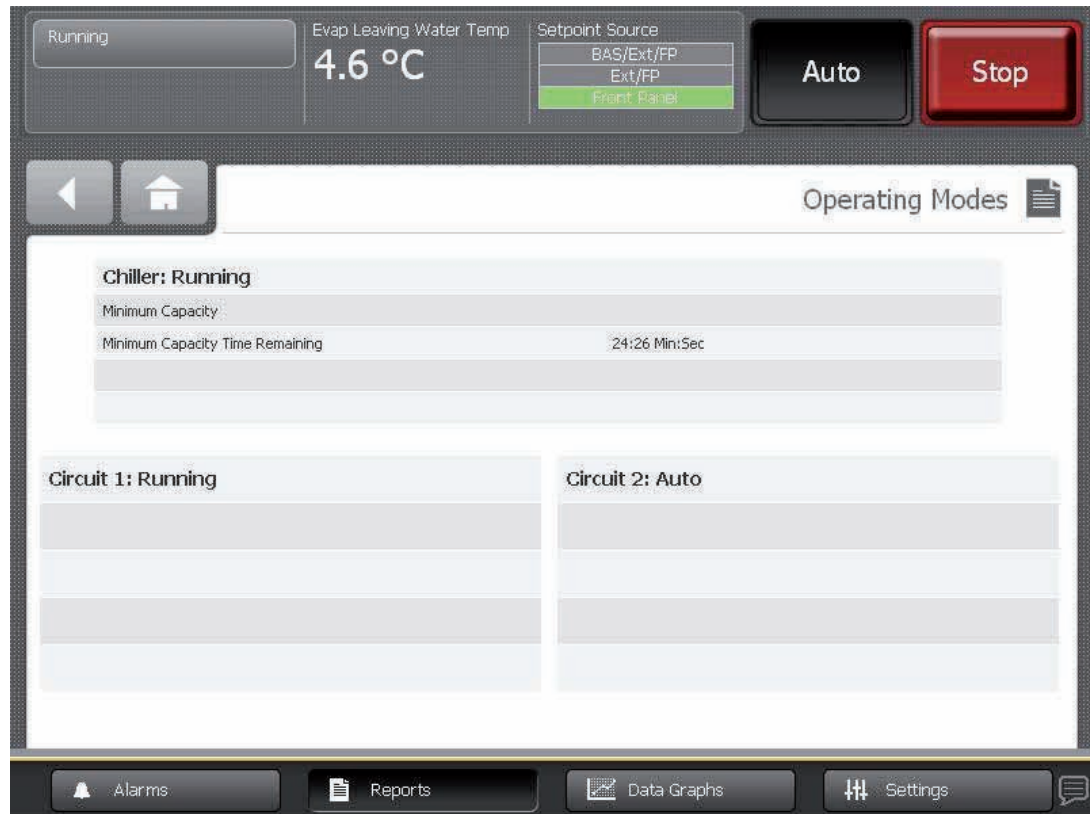
Figure 12. Chiller Operating Modes screen for Duplex CDHF and CDHG chillers
