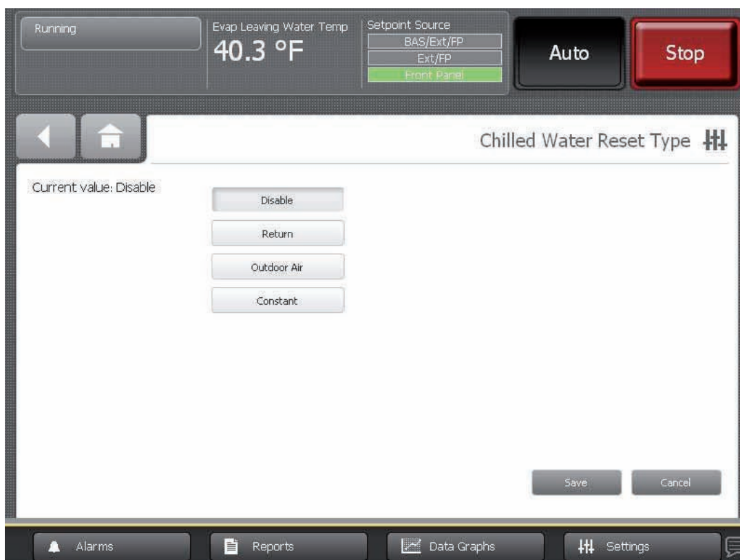
Figure 22. Example equipment settings screen with buttons for changing setting
