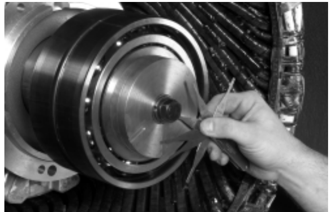
Figure 39. After applying torque with an impact wrench to the cap screw, measure the gap of the direct tension indicator and hardened washer in all 5 places. The average of all gaps must be .015" to .020", with no individual gap greater than .025" or less than .010". If a gap is greater than .025", tighten again using the impact wrench and repeat the measurement. If a gap falls below .010", remove the cap screw and washers and install a new KIT07314. Repeat the above procedure.
