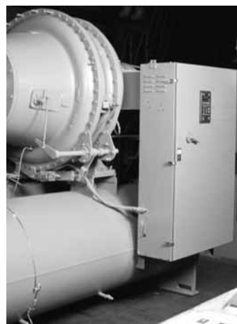
Figure 19. Unit mounted starter
