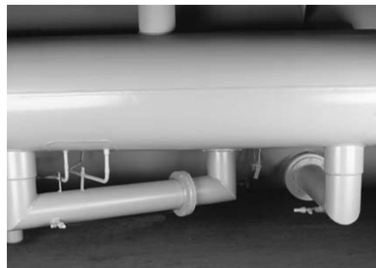
Figure 17. Condenser liquid line flange
