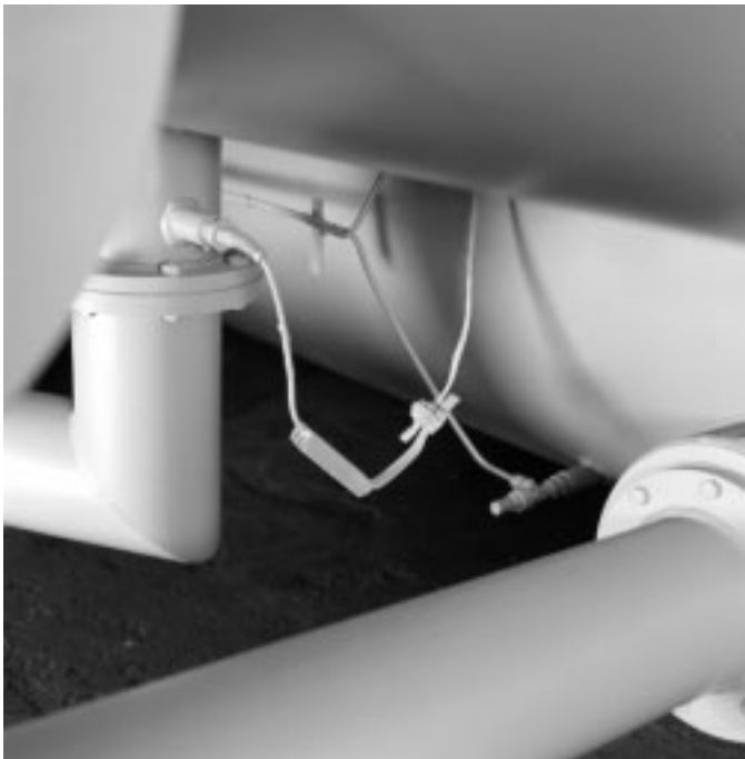
Figure 18. Evaporator liquid line flange
