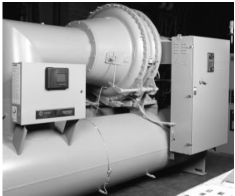
Figure 21. Unit mounted starter
