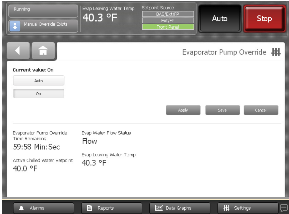
Figure 27. Manual Control Settings screen (Evaporator Pump Override shown)
