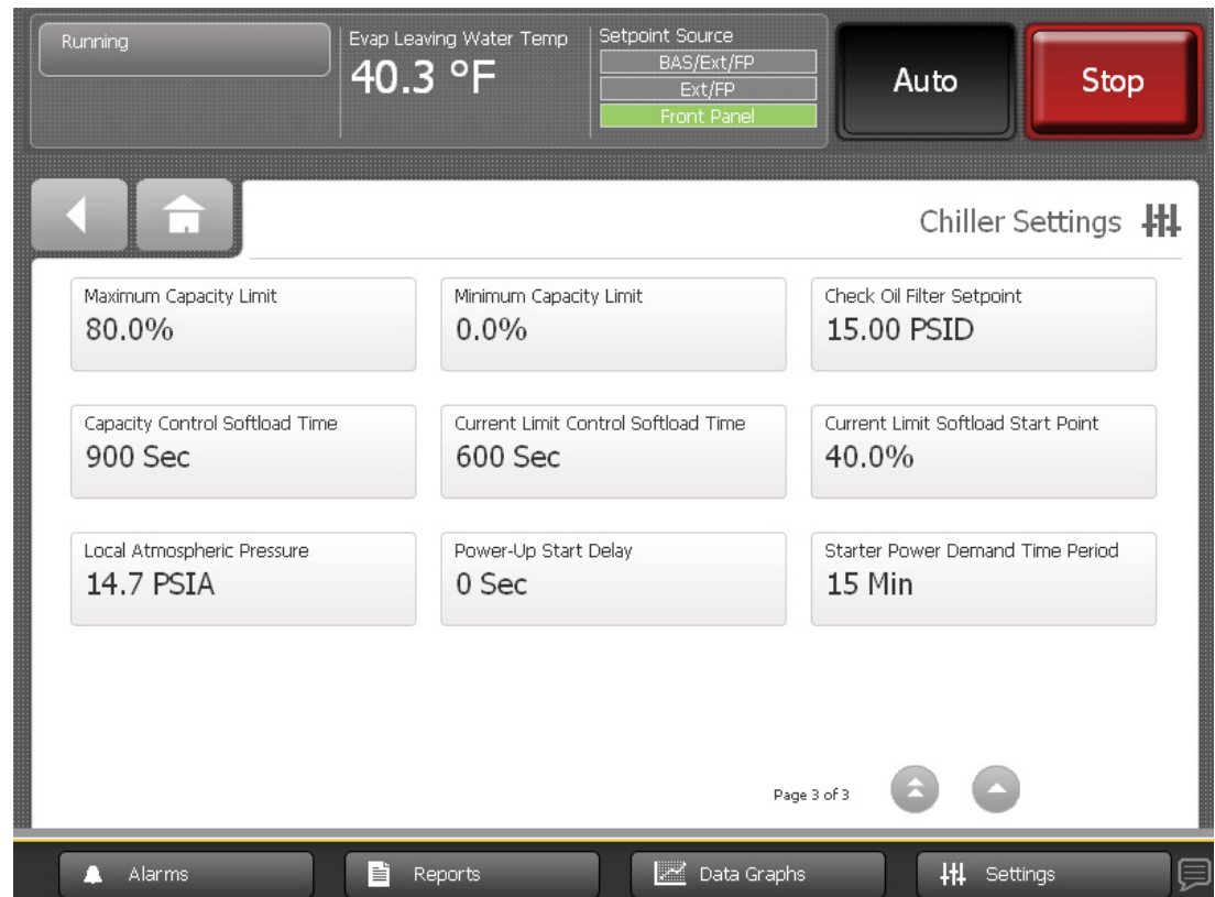
Figure 21. Example equipment settings screen (Chiller Settings shown)
