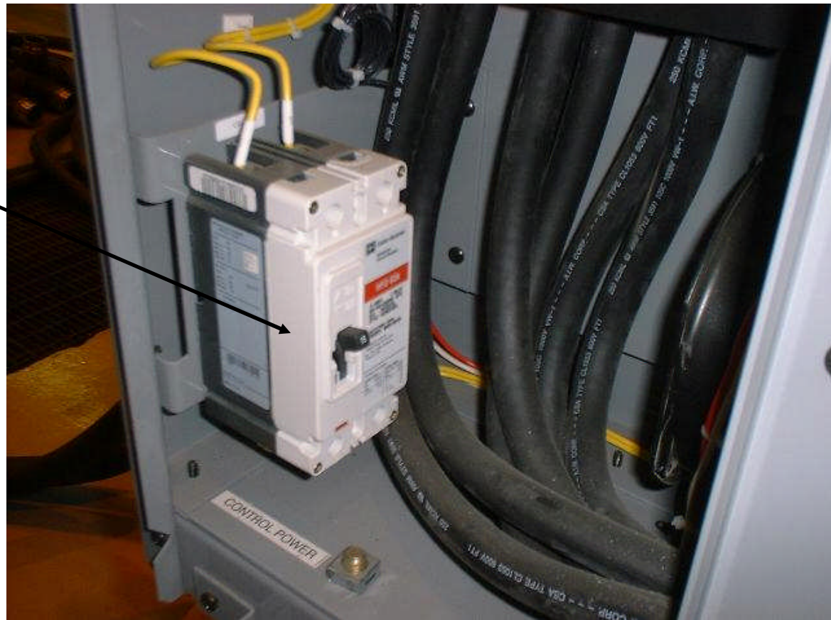
Control Power Circuit Breaker
