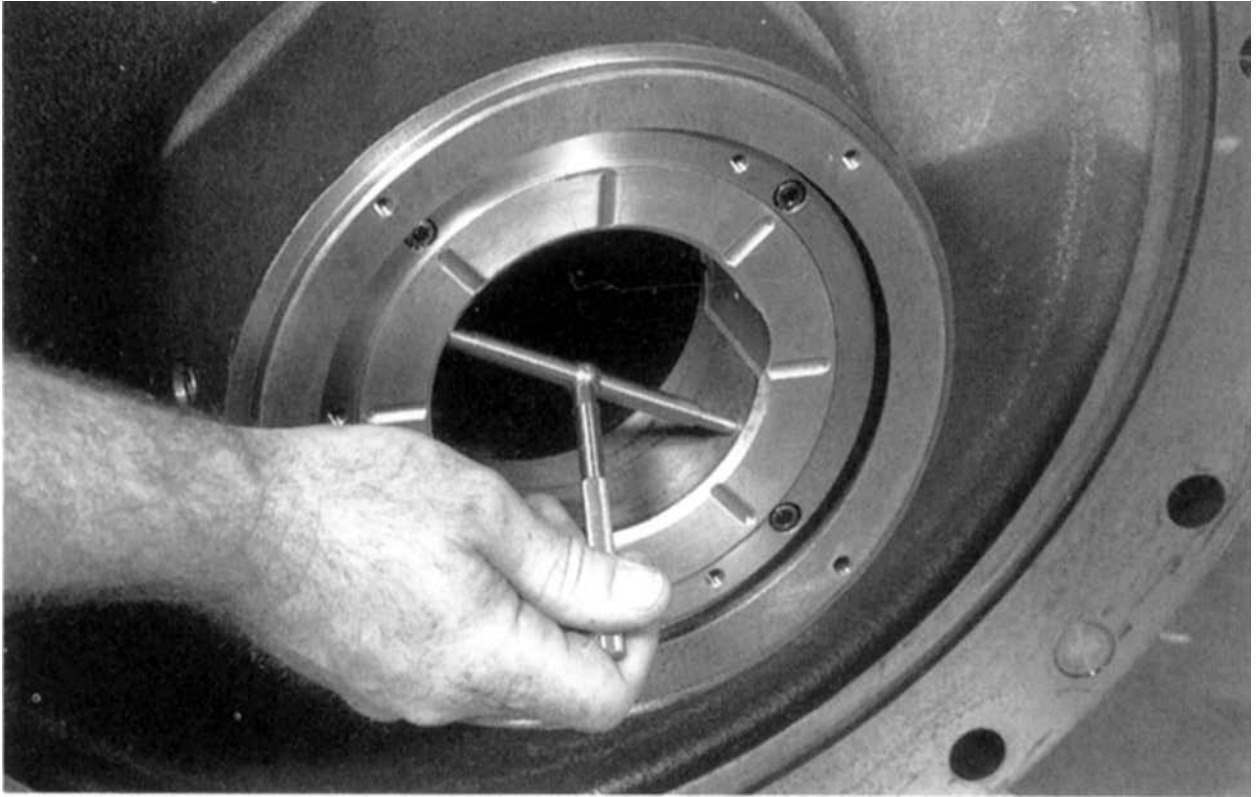
Figure 53 — Measuring the Drive End Bearing
