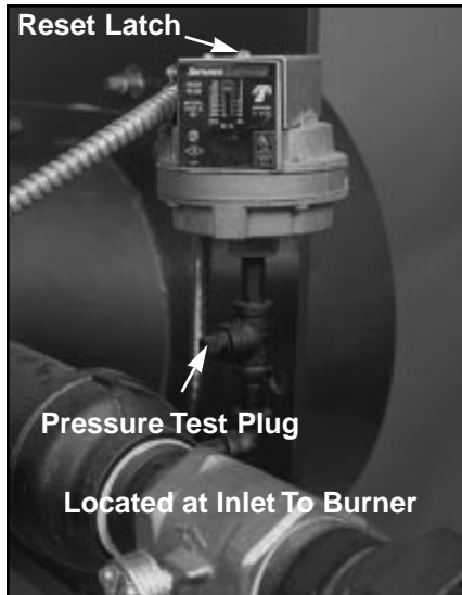
Fig. B15 High Gas Pressure Switch
