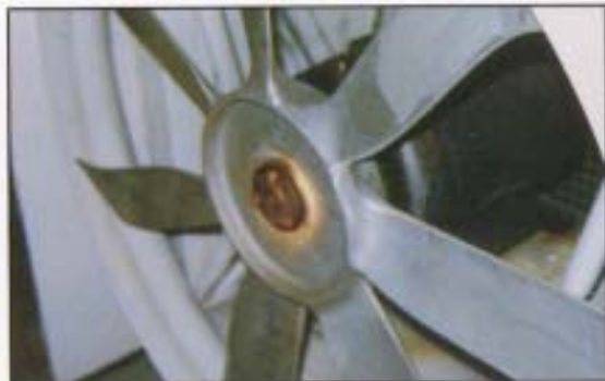
The addition of SO_2 to the grape storage environment visibly corrodes the galvanized fasteners on the fan hub, while leaving the aluminum blades intact.
