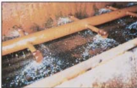
The results of inadequate water treatment are displayed on the surfaces of this galvanized steel coil.
