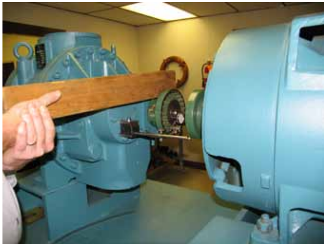
Figure 2 Board is positioned between the compressor and coupling to force the rotor towards the motor.
