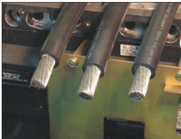
Figure 20 - Insulation Stripped from Power Leads
