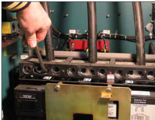
Figure 21 - Fastening Power Leads
