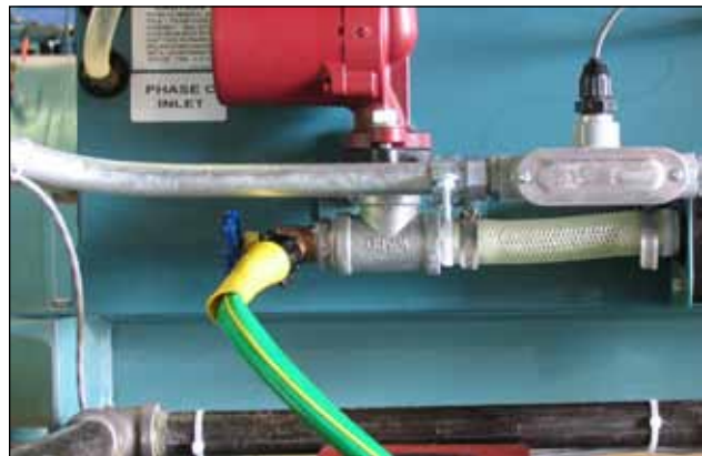
Figure 34 - Hose connected to the Heat Exchanger Drain
