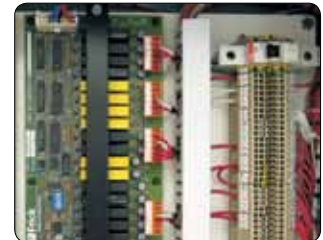
Circuit Breaker Protection for Main Power
