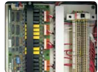
Circuit Breaker Protection for Main Power
