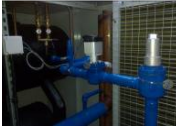
Capped stop valve to the right of the photo with the control actuator to the left
