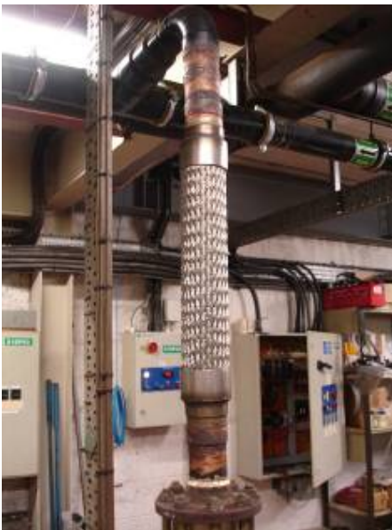
Incorrectly installed vibration eliminator
