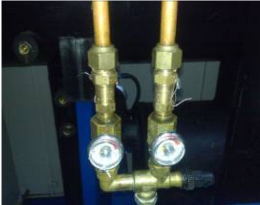
An example of good practice in pipework
