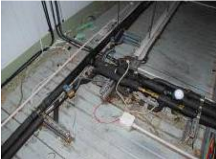
Poorly laid out pipework on the ceiling void of a chill store
