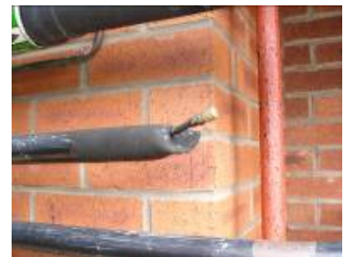
A Schrader badly fitted into the end of a poorly sealed copper pipe
