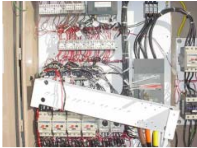
FIG. 4 - FUSE PANEL REMOVED
