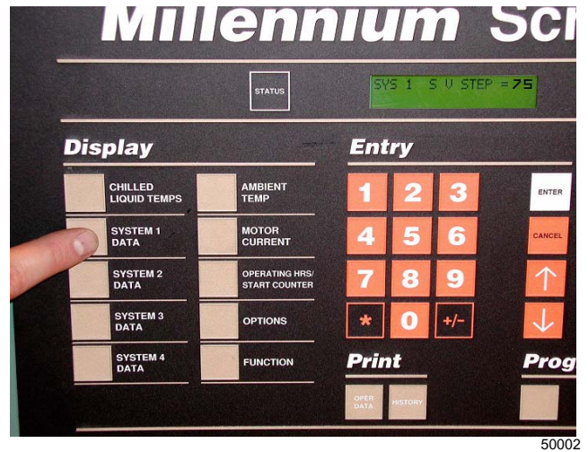
FIG. 1 - Run Compressor to Full 75 Steps
