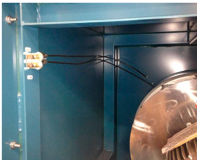
FIGURE 12 - HIGH AND LOW CONNECTIONS AND ASSOCIATED TUBING FOR FAN MOUNTED AIR MONITORING SYSTEM
