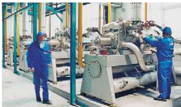
Example of a Unisafe ammonia application
