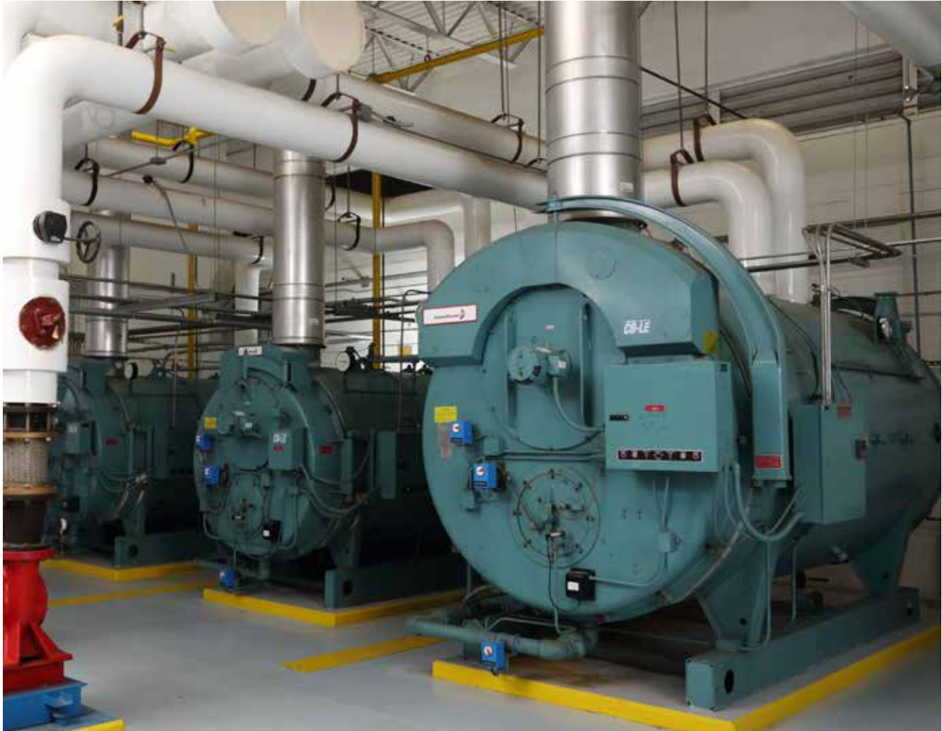
Figure 1-11: Operational Boiler Room
